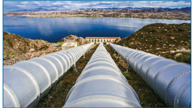
Whitsett Intake Pumping Plant on the Colorado River.
